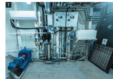
1 Drylab 2 Ferrybox 3 Deep Trekker Revolution 4 Mini SVS 5 Weather station 6 Sims 7 Underway system.
